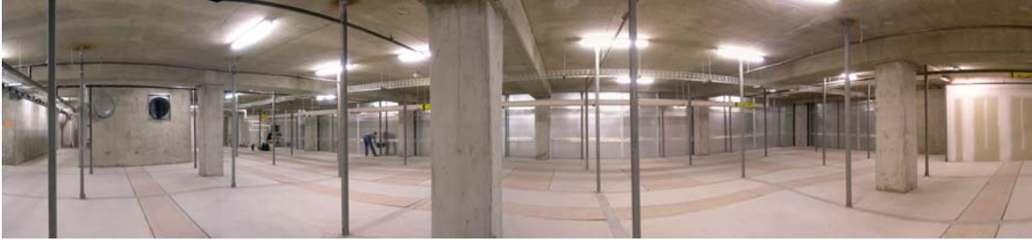
Illustration 7: Building 4; Panoramic view of ceiling space, measurement in progress along curtain wall in background.
