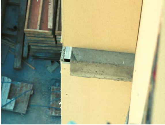
Illustration 1: Walls and supporting slab misaligned; on one side the slab projects from the wall sheathing, on the other it's retracted. The same detail applies to both—the designer envisioned the slab edge and face of sheathing in alignment.
